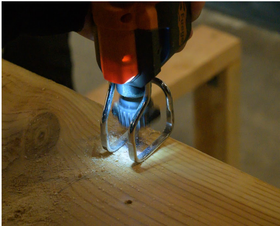
Figure 24: A close-up shot of the cutting of the device's vertical wood boards.
